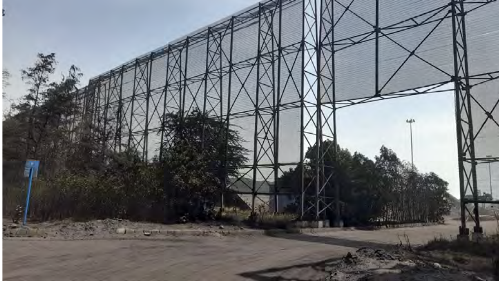
Installed Wind Screen
