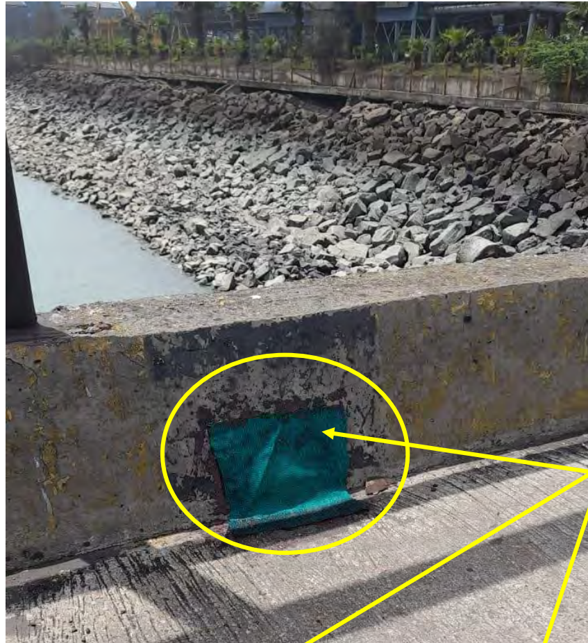
Filters at Jetty Outlet
