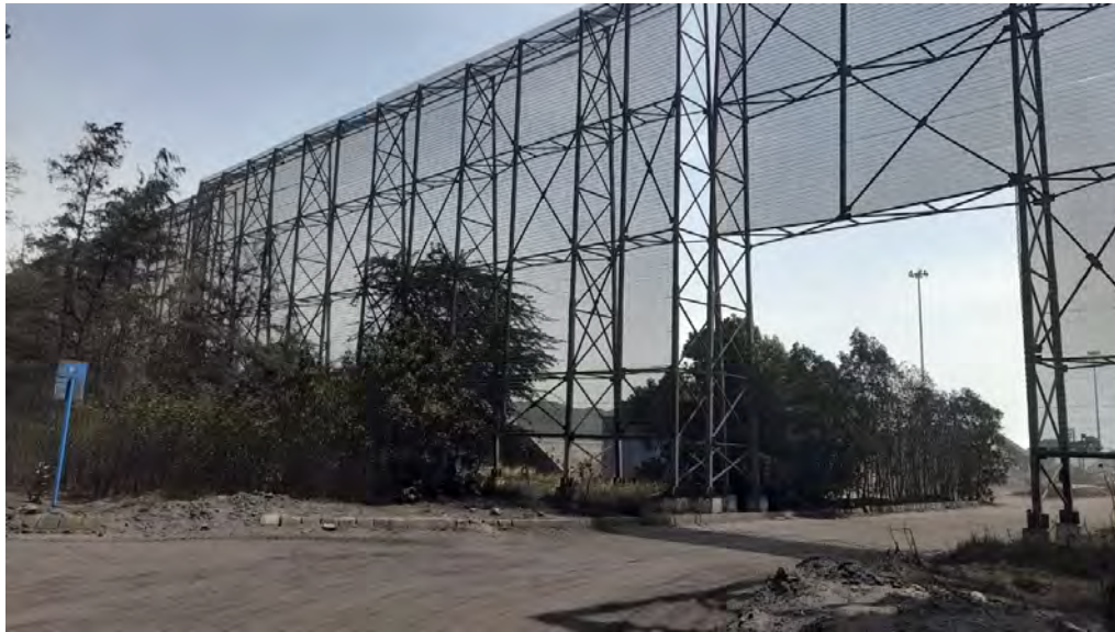
Installed Wind Screen
