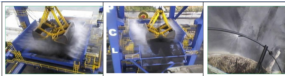
Figure 2:3 Mechanical Dust Suppression System at Ship Un loaders using Sprinklers system
