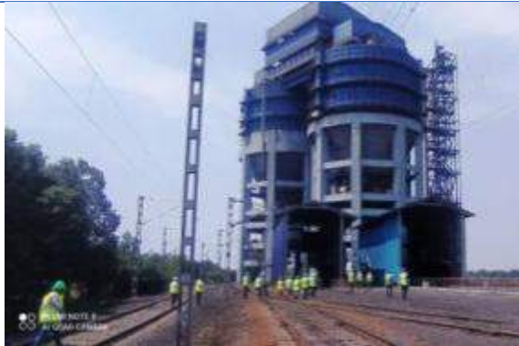
Silo for Railway rake loading
