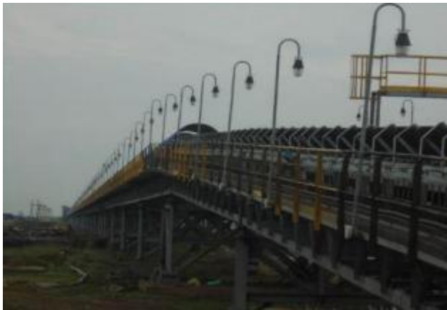
Conveyor Systems directly transferring cargo to industries
