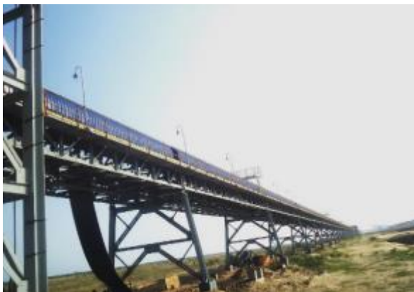
Closed Conveyor system
